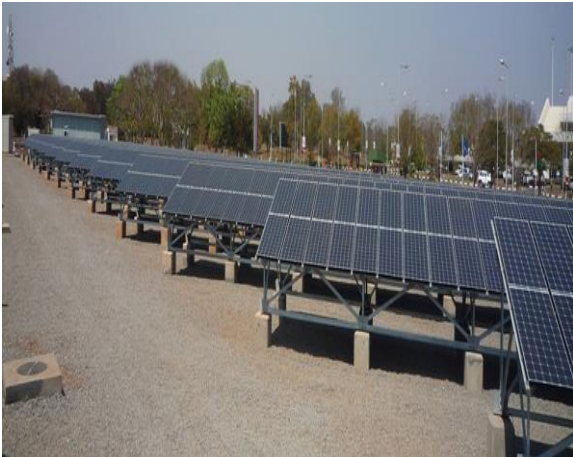
Grid connected Solar PV Farm at Kamuzu International Airport
