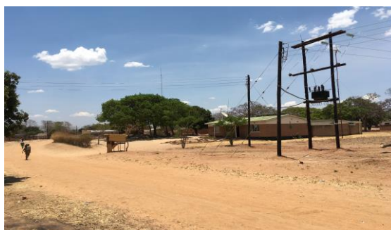
Distribution transformer supplying customers
