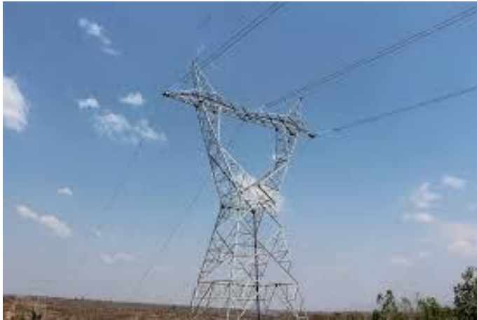
Figure 2:400 kV transmission line
