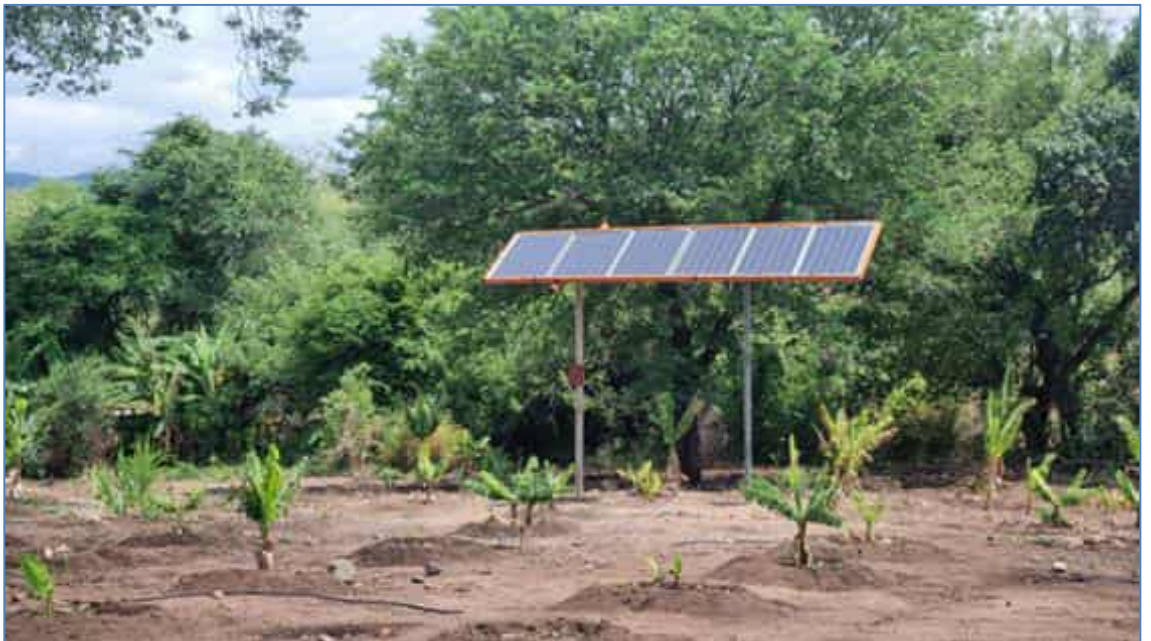
Figure 79: Solar panel that powers four water sprayers to irrigate the crops at Titani Ranch
