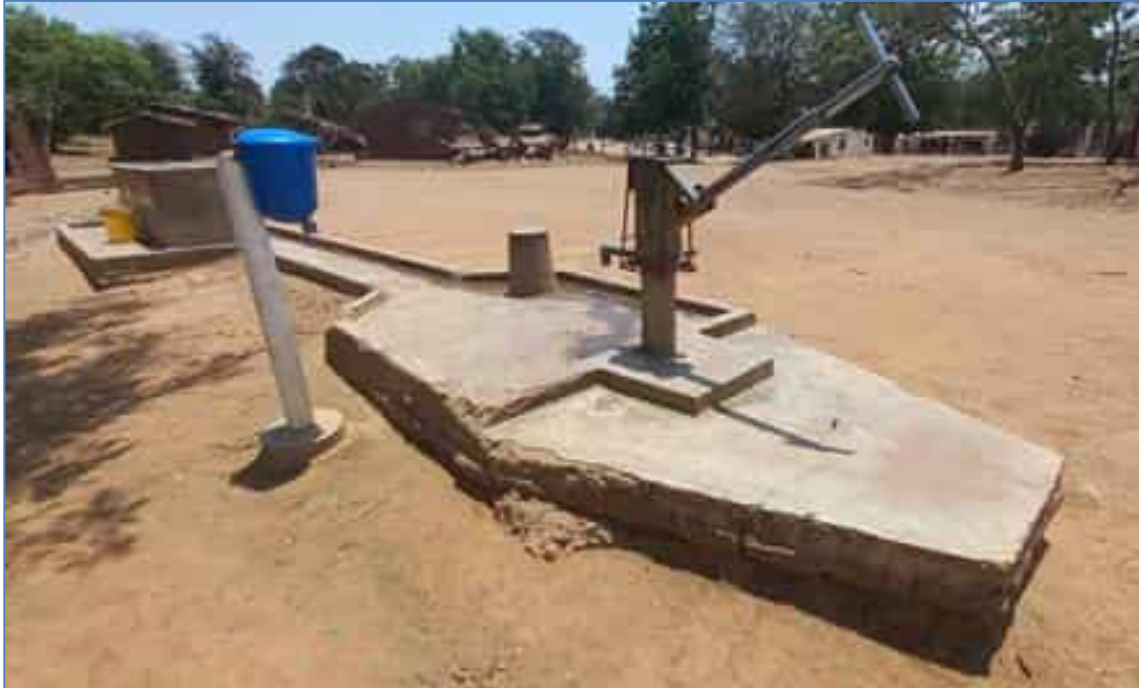
Borehole with Chlorine Dispenser
